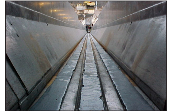
Chute protected with ARC BX1*
